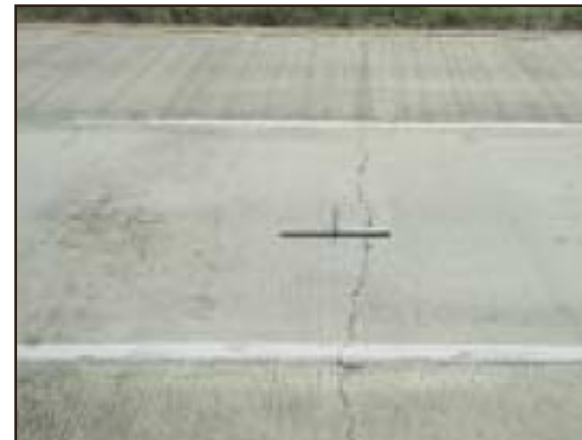
Moderate Severity Transverse Cracking
