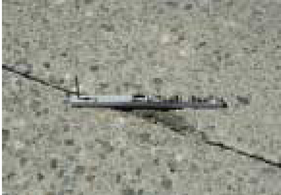
Moderate Severity Spalling
