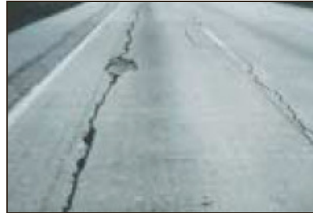
High Severity Longitudinal Cracking
